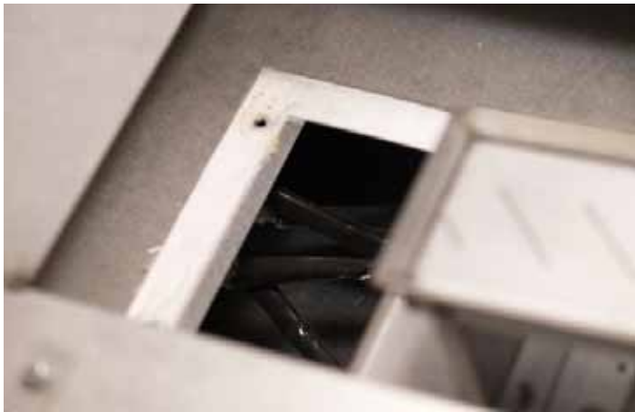
Figure A1 - Halcyon Burner Moved To Right Revealing Connections
